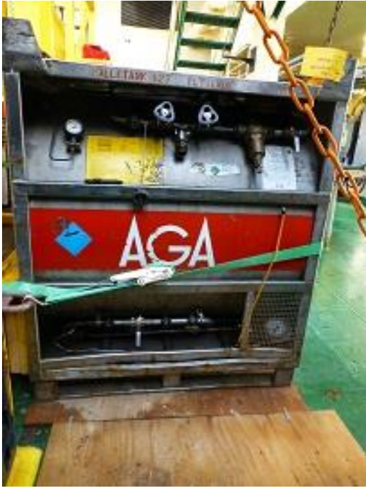
The type of pressurized LN2 tank delivered by AGA, that did not meet the specifications for loss by evaporation.
