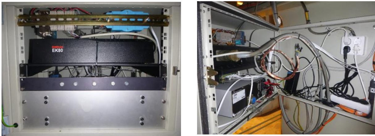
Figure WC-3: EK80 WBT installed in rack with EK60 GPT in tween deck below gym. Left – front view of rack with front door open – GPT is behind gray panel on bottom. Right – back view with back door open – GPT on lower level – WBT on upper level.
